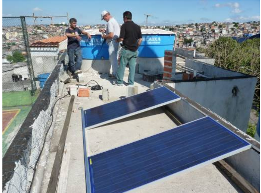
The system integrator uses CX40 charge controller for reliable power supply for a school's IT infrastructure and for its back-up system
